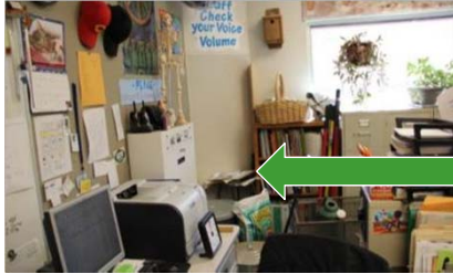
Diffusers blocked with clutter and posters!
