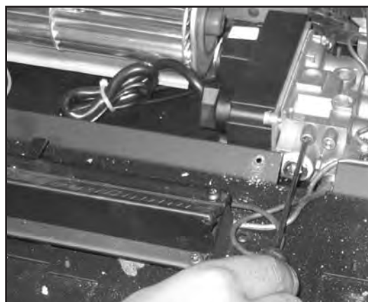
Figure 52: Opening Inlet Pressure Tap on Valve.
