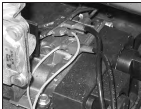
Figure 35: Spill Switch Wires Connect to Thermocouple.
