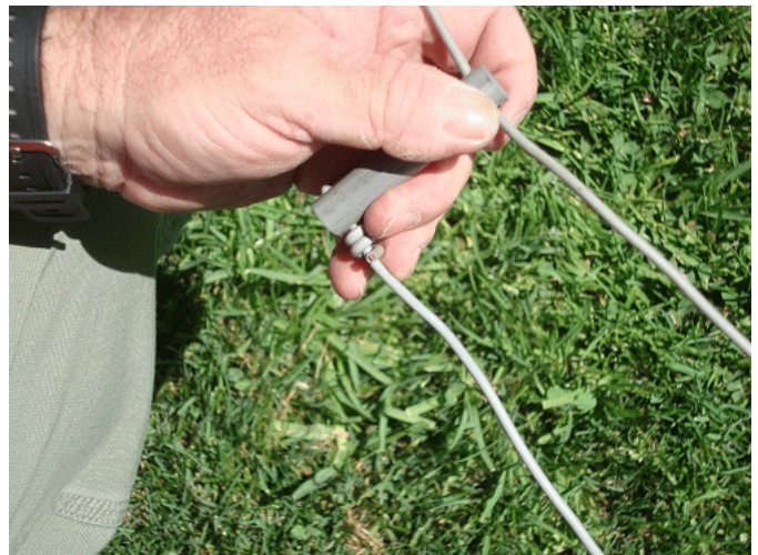
Closeups of spacers between band conductors.
