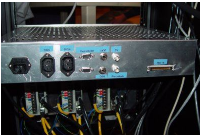
Figure 8. View of the rear of the rack-mount enclosure housing the predecessor of the 1902 board. From the left: one 120VAC receptacle, two 120VAC sockets, hygrometer “D” connector, Unused “D” connector, gas solenoid power jacks, 5VDC supply for the droplet detector laser, 5VDC BNC for the the droplet detector photodiode, and 68-pin interface board connector.
