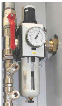
Compressed air supply
