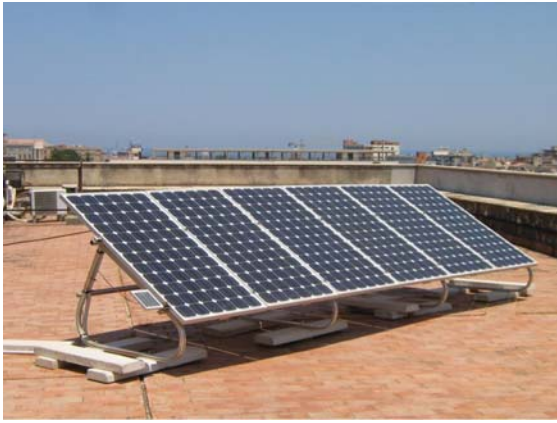
Figure 3: The string picture of the PV system
