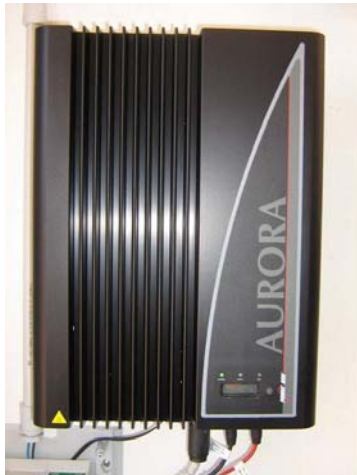
Figure 4: The PV system static power converter
