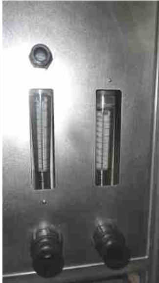
Plumbing Manifold and Flow Meter connections
