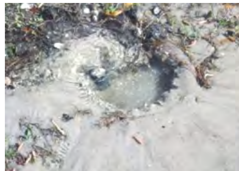
Broken piping underground causing puddling and erosion
