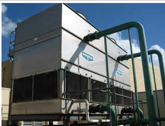
A clean and well-maintained cooling tower
