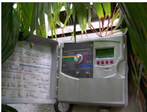
Figure 59. A smart irrigation system control box.
