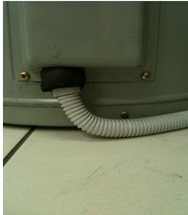
Figure 1. 20mm corrugated plastic conduit cable entry into the terminal box with Armaflex sealant to terminal box lid.
