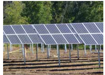
A completed section of the solar array in Caro.
