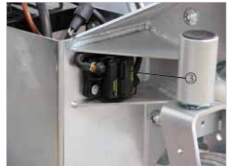
Fig. 78: Main safety switch
