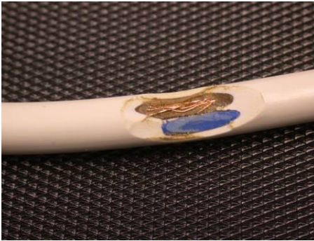
Damage to power cable sheath.
