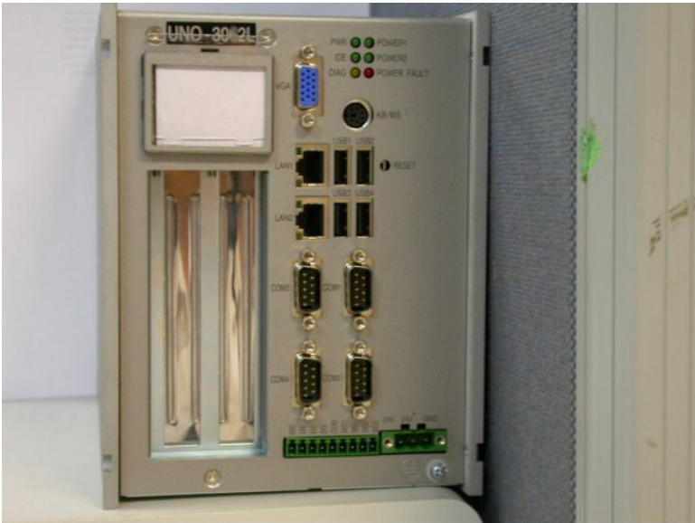
Figure 3.6: UNO-3072L Improper Installation (2)
