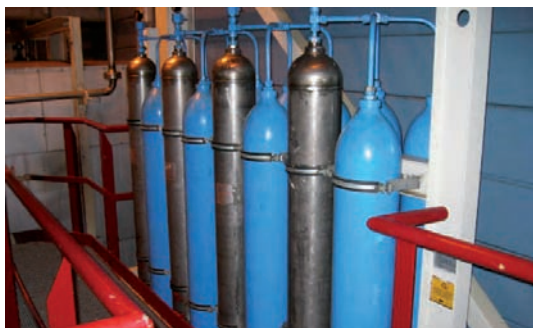
Storage rack with bolted cylinder brackets
