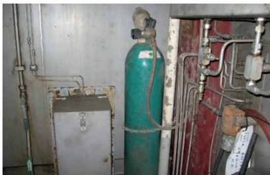
Temporary storage, secured with chain
