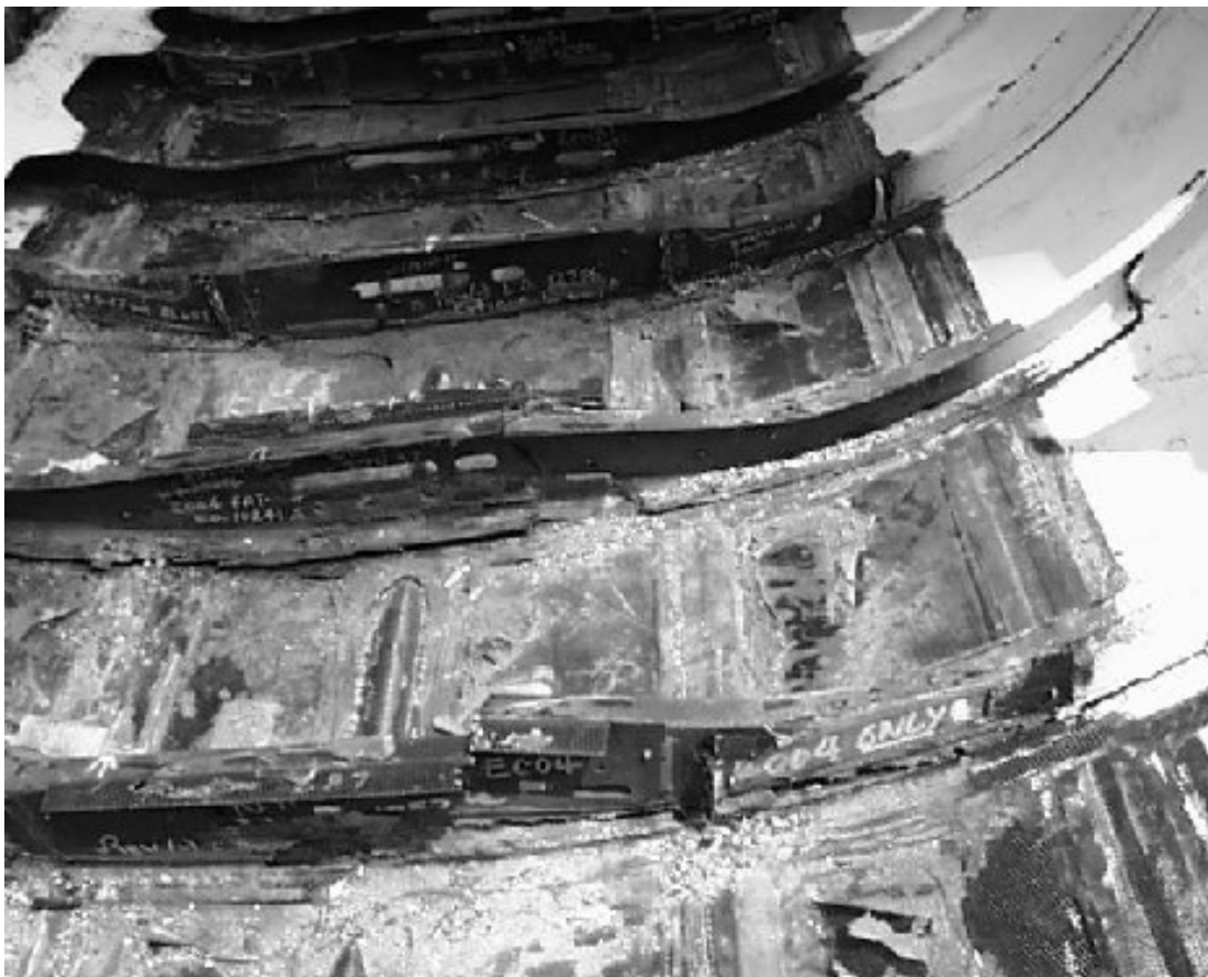
Figure C-4. Photograph showing interior damage and frame failure.
