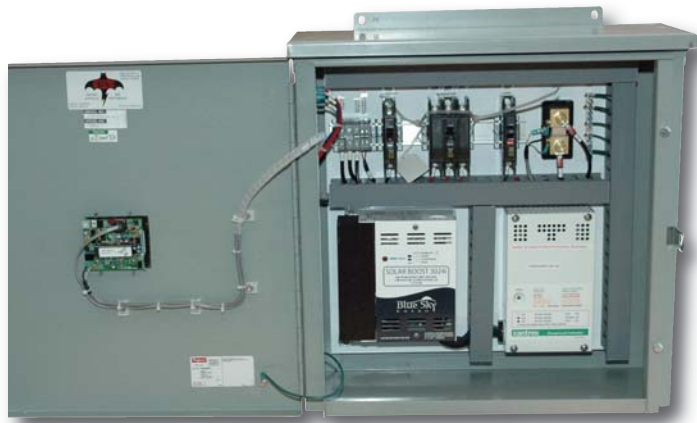
Figure 2-20 - DC Charge Controller Display with Low Voltage Disconnect and Circuit Breakers
