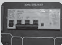
Fig.13 30mA leakage breaker Three phase off
