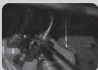
Fig.15 air purge over fuel injection pump
