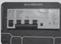
Fig.13 30mA leakage breaker Three phase off
