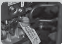
Fig.16 oil dipstick on diesel engine
