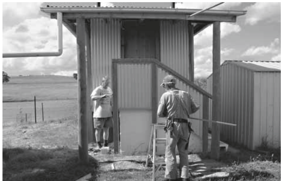
A couple of mates helped with the balustrade – on the left is Monty who came over from England for three weeks just to help me build!
