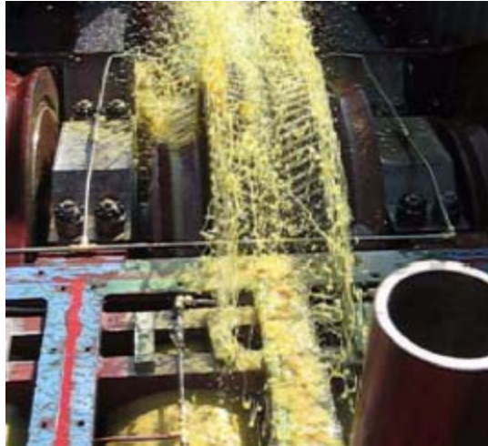
Fig. 2-2 Oil Splash when Pump Operates
