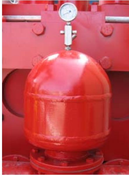
Figure 6-3 Suction Desurger & Pressure Gauge
