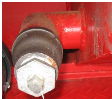
Figure 6-1 Liner rinsing system drain
