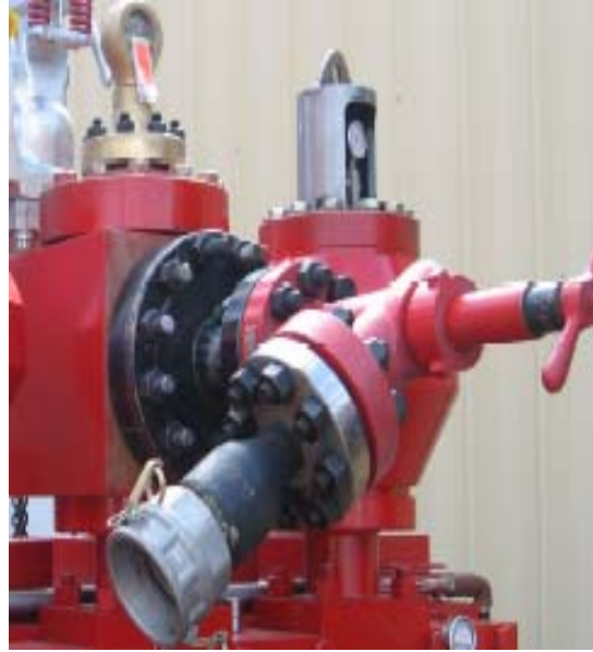
Figure 6-5 Strainer Cross with Choke valve
