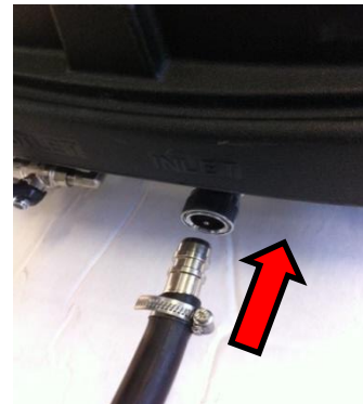
Fig.15 – Mains supply water inlet
