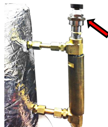
Fig. 19 – Water probe sensor and boiler level gauge
