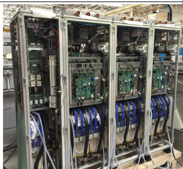
Multi terminal PED (doors removed)
