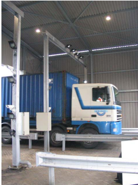
Photo 3.4.1: SeeGate 2 Installation (Rotterdam, The Netherlands)
