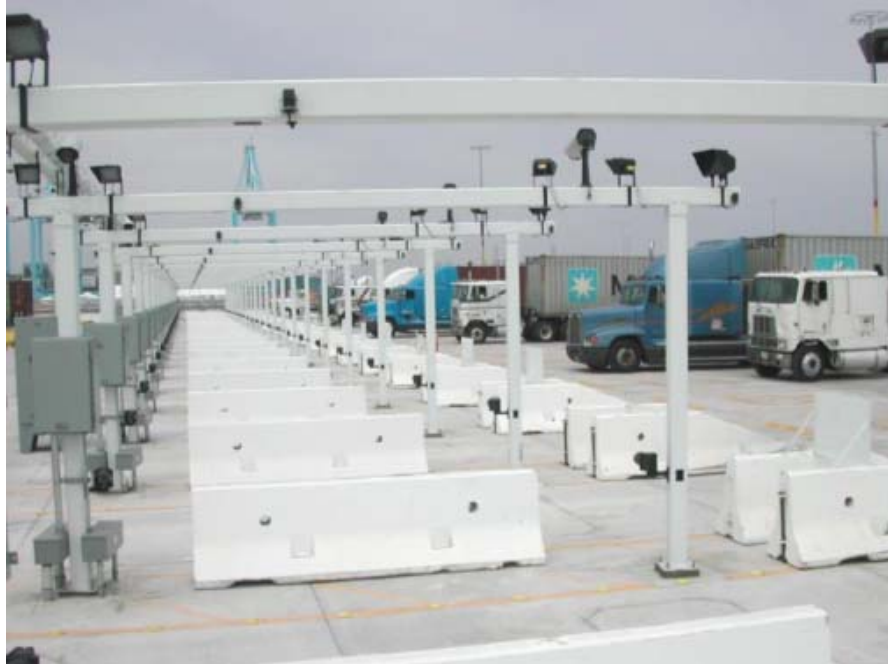
Photo 3.4.4: SeeGate 1 Installation – APM Pier 400 (LA, California)
