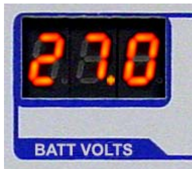
Fig. 11. Voltage readout/Test panel.
