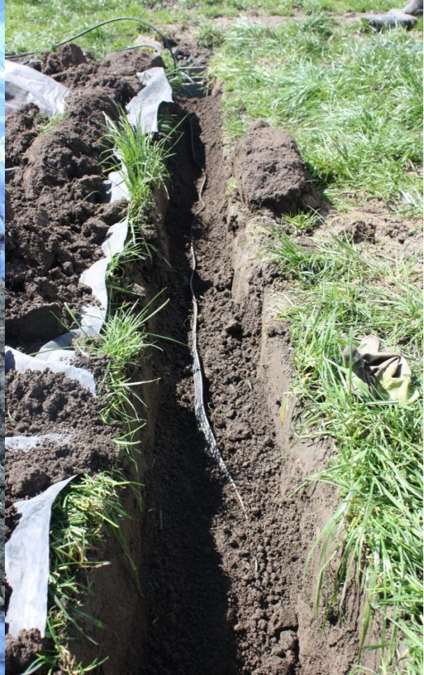
Top sensor installed to 250mm at the deep end.
