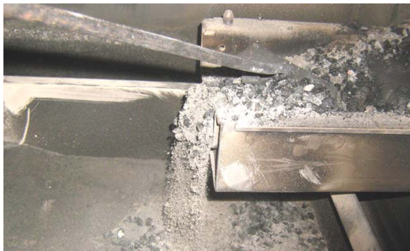
Figure 2.12. Ash and char cleaning procedure of the material, laid on the burner's grate;
