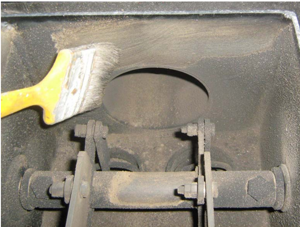
Figure 2.5. Cleaning the ash deposits off the heat exchanger surfaces, as well as off the ash cleaning mechanism;
