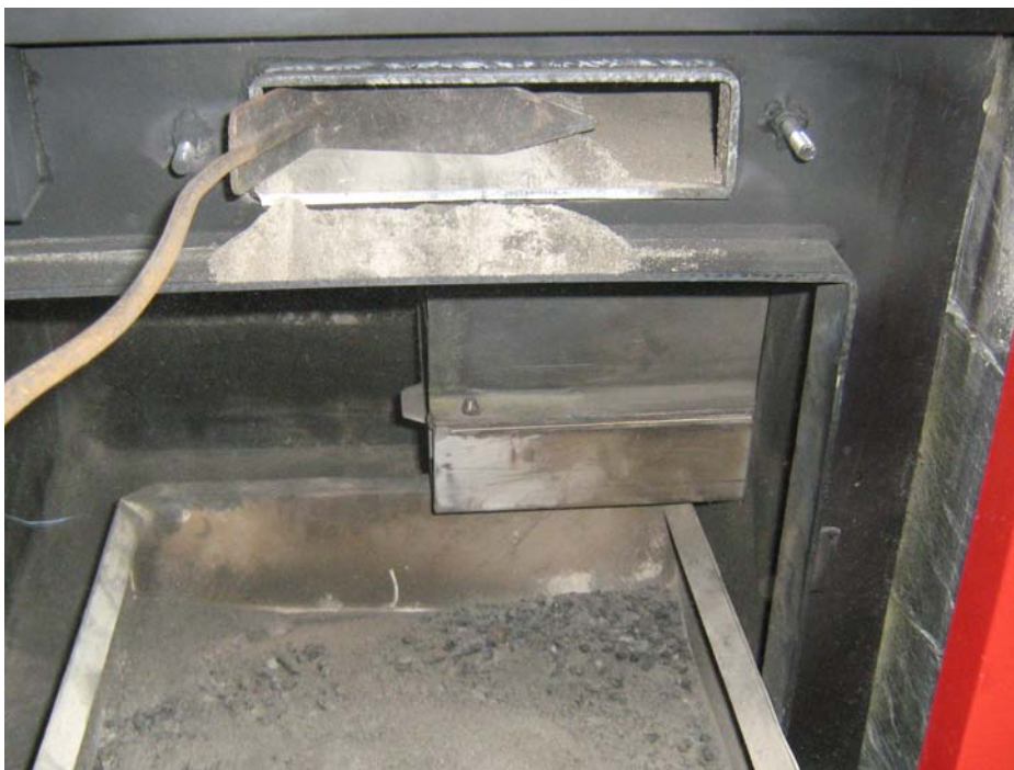
Figure 2.10. Cleaning of the ash in the secondary deposition zone of the heat exchanger (right beneath the pipes of the heat exchanger);
