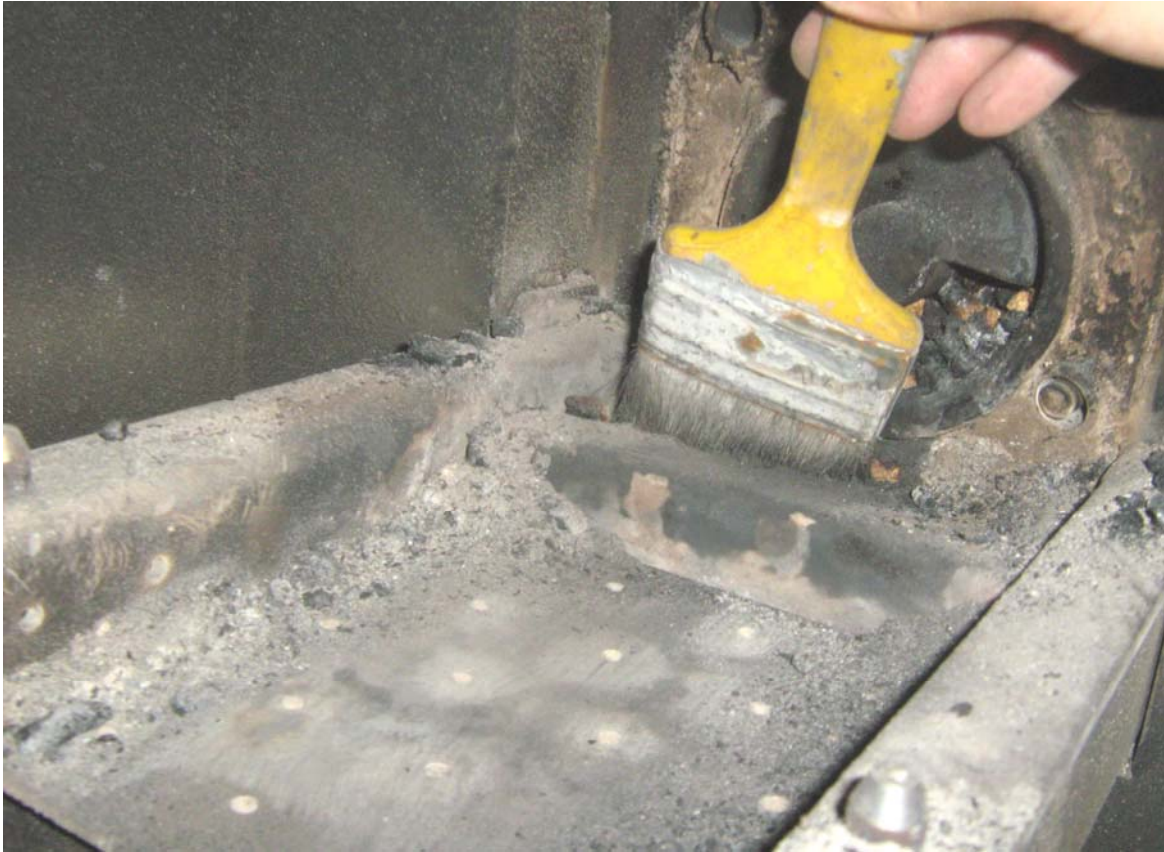
Figure 2.13. Brushing and cleaning the ash residue and any other char remaining on the burner's grate;
