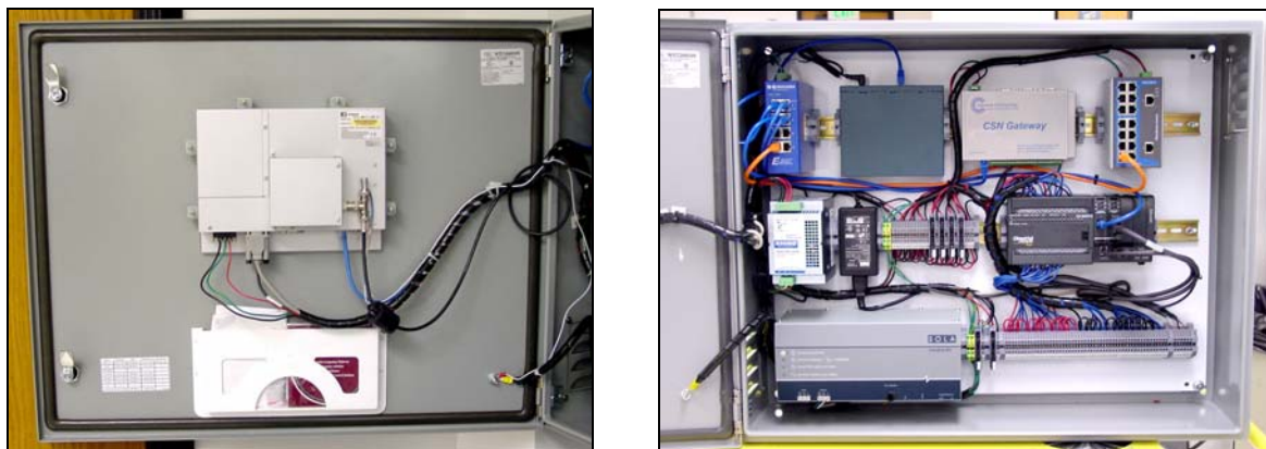
Figure 1. Internal Views of an APS-115-C001 with Remote Monitoring Hardware
