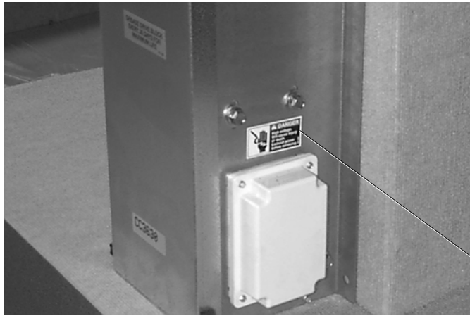
Decal-889 is located above the electrical box on the outside of the Curtain Controller
