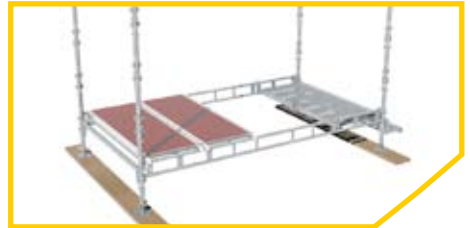
8 Install Entrance step and check for square using the erection platforms and the Landing Platform
