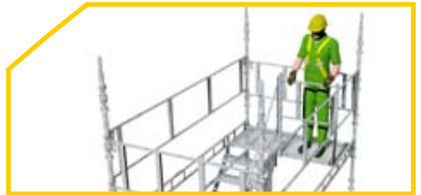
26 Temporarily fit Guard Frame to protect upper platform. This may be moved up as the stair tower progresses.
