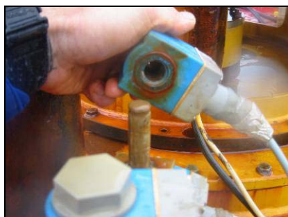
Fig. 4.4 Saltwater corrosion of solenoid (23.06.03)
