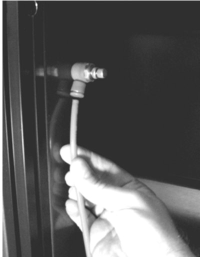
(Figure 3-4 Air compressor valve)
