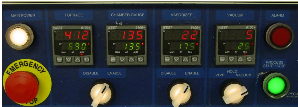
Figure 9. Front panel switches and buttons and process controller readouts. Red numbers (top) are actual readings; Green numbers (bottom) are set point values.
