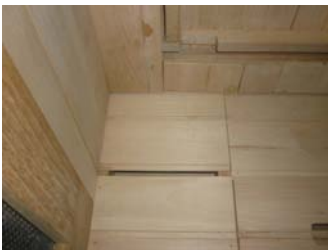
Front floor electrical cover
