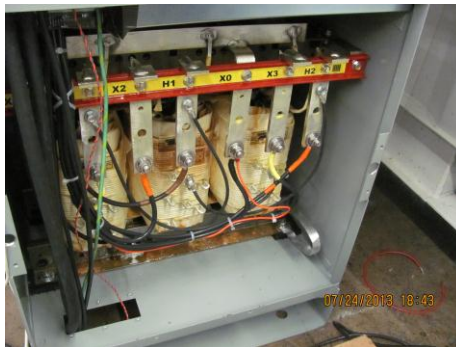
Figure 16: Position of the internal isolation transformer in the GTIB-30 enclosure.
