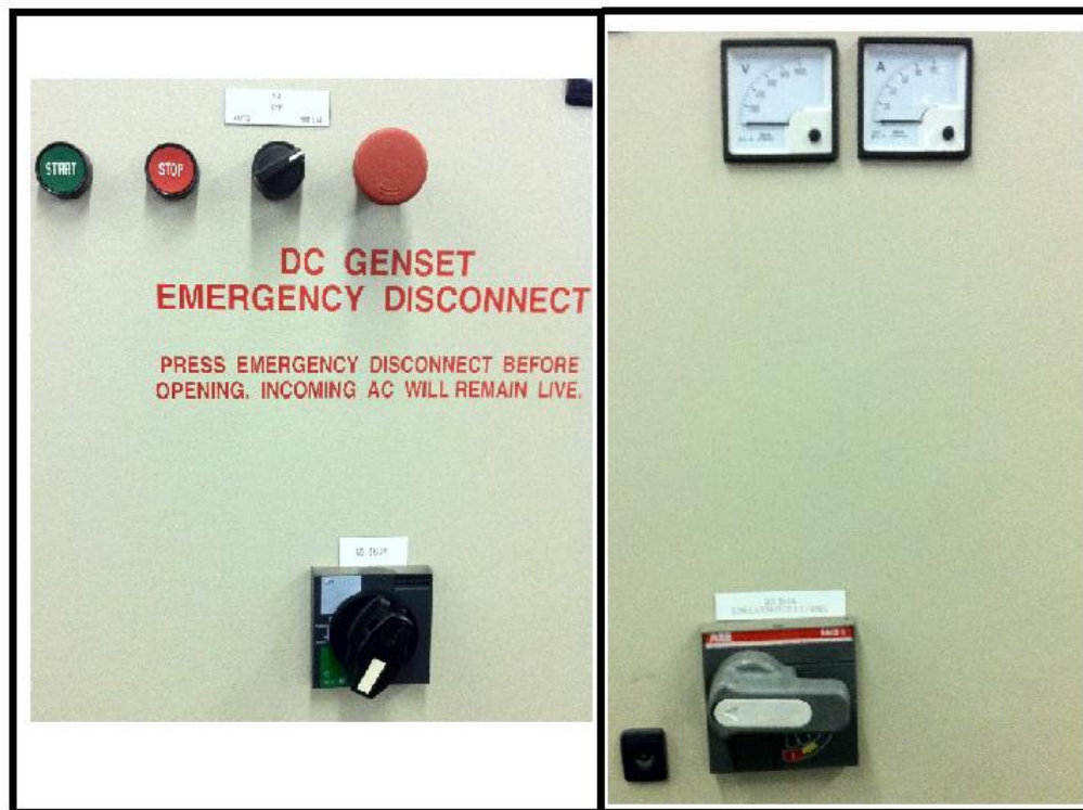
Figure 11 - DC Genset AC circuit breaker(Left) and DC Genset DC circuit breaker (Right)
