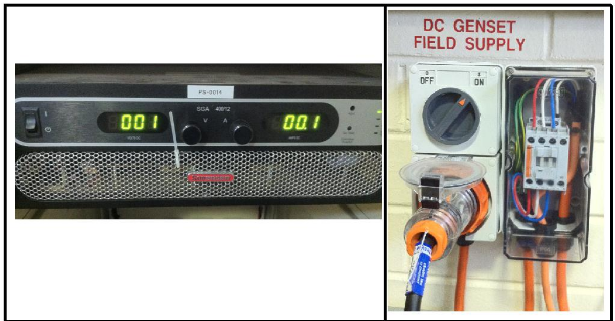
Figure 9 - The Field Power Supply (Left) and the DC GENSET FIELD SUPPLY output (Right)
