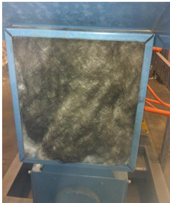
Figure 12 - DC genset air filter
