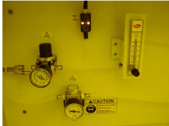
Figure 10. Lower pneumatic panel.
