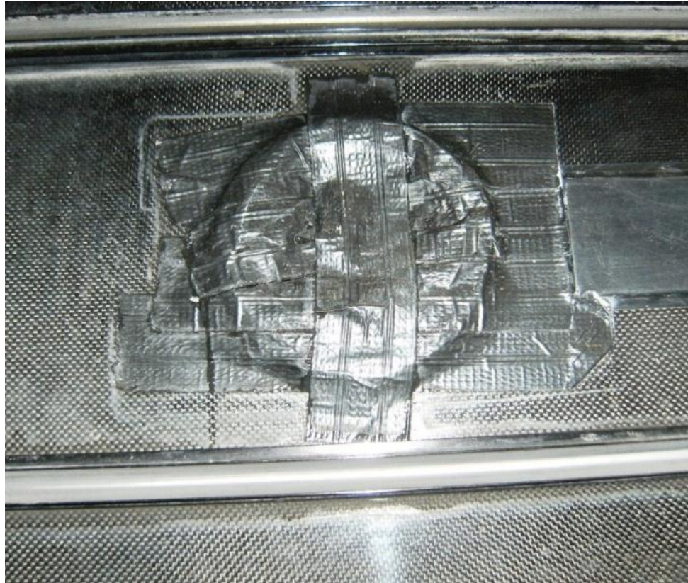
Hatch cover only taped over – Not Acceptable
