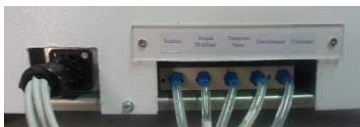
Picture 1. 2 – Connections of probes on the external level
