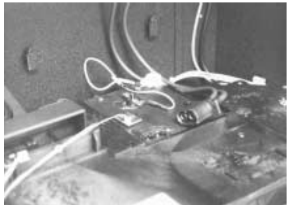
Lamp connector disconnected
