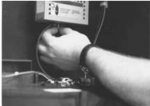
Loosening screw at bottom of ballast
