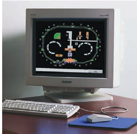
Perimeter Monitor (Operator Graphic Display)
