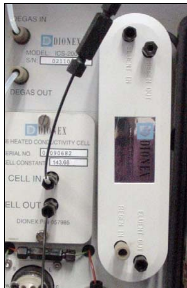
Figure B-21. Suppressor Installed (SRS Shown)
