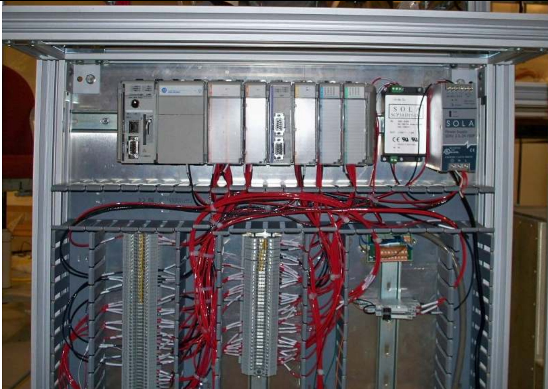
Figure 3.5. Panduit DIN rail with wiring.
