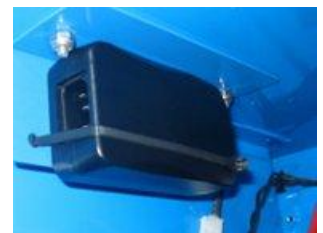
Fig. 4: Lighting power supply
