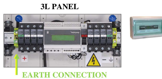
(2) ESP PANEL EARTH CONNECTION
