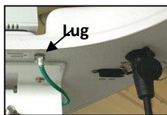
Figure 28: The ground lug connected to the bottom of the WeatherHawk.
