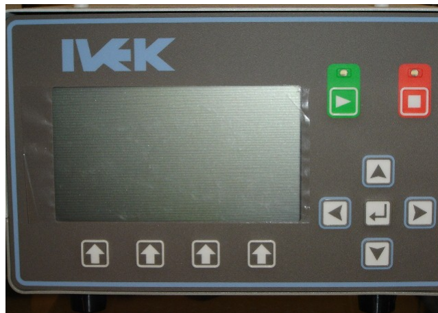
1 of 2 IVEK Spray Controllers
