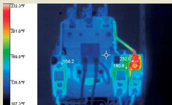
Hot connection, pump
