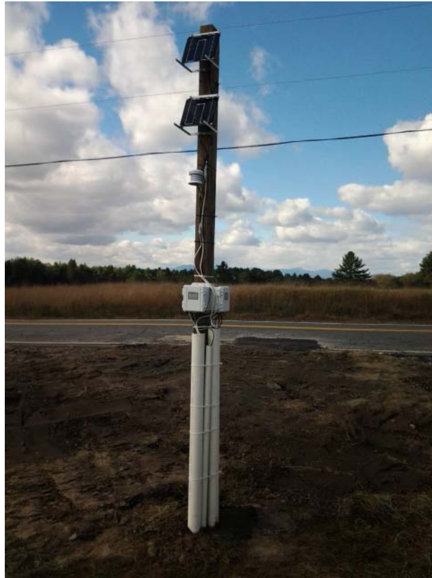
Figure 3: An example of a completed deployment cellular transmission site.
