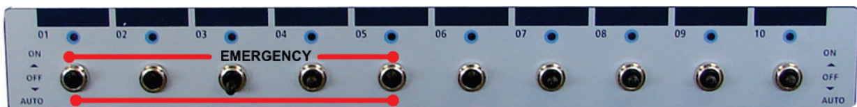
Figure 3: Emergency Relay Switches
