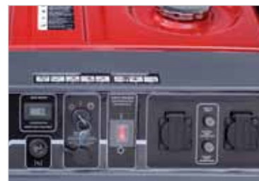
Dashboard including hourmeter, engine controls and circuit breaker.
