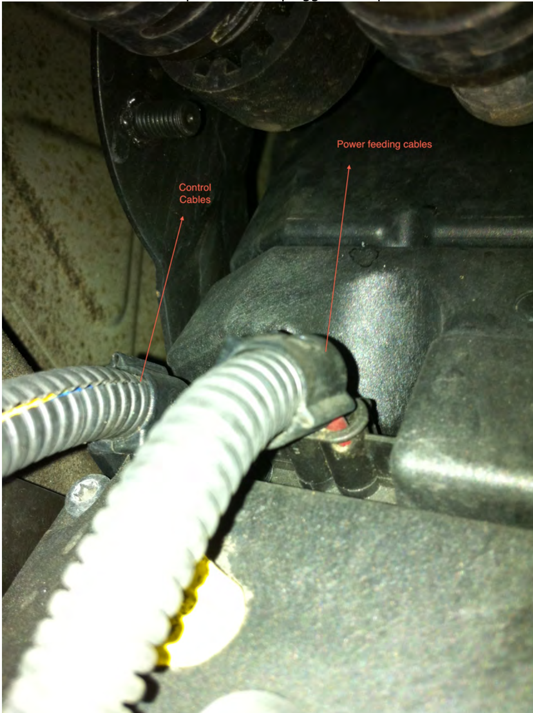
Picture 13 – Control and power cables plugged on top of the heater.
